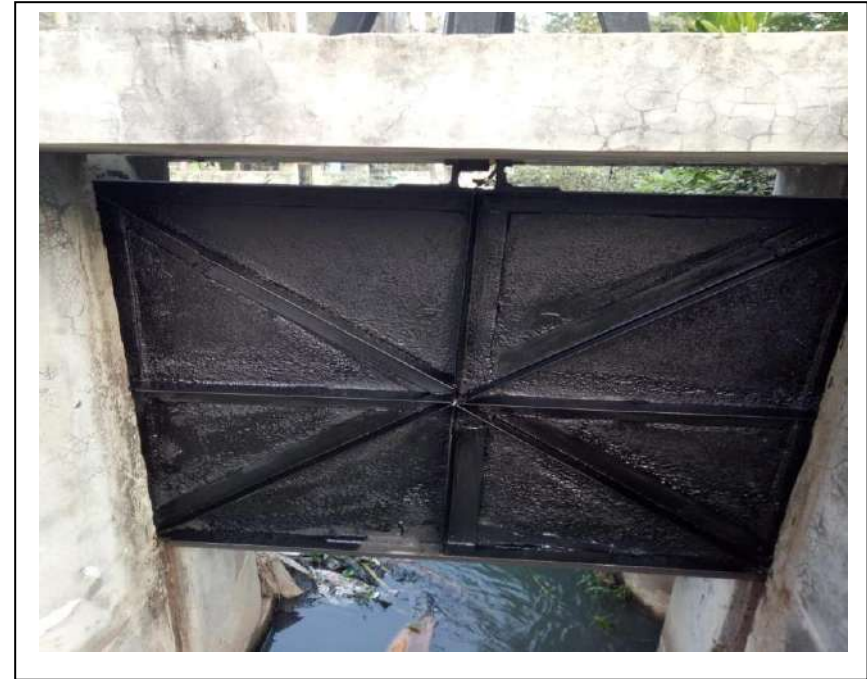
HALISAHAR DRAIN LOCKGATE
