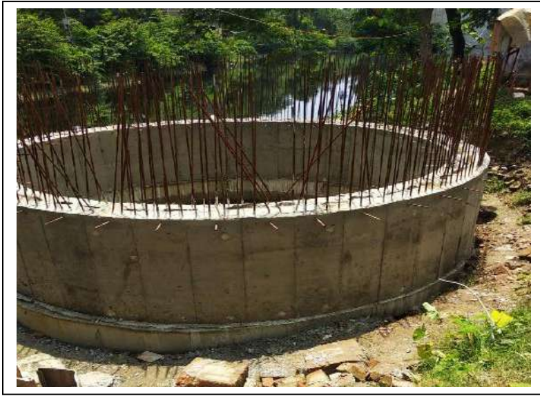
LIFTING STATION-7, BUDGE BUDGE
