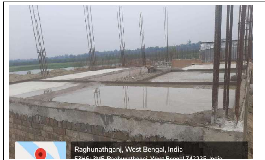
CHLORINATION -RAGHUNATHGANJ STP
