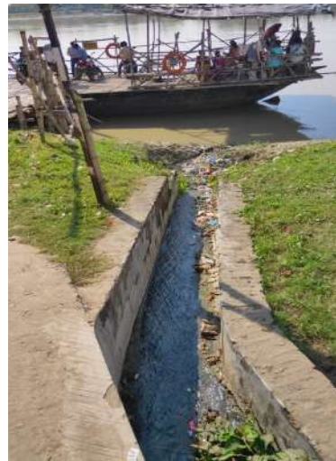
Outfall falling into Ganga
