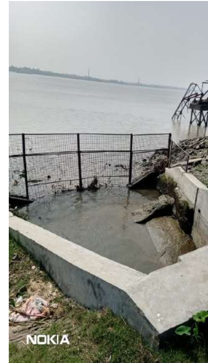
Outfall falling into Ganga
