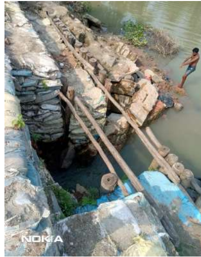
Outfall falling into Ganga
