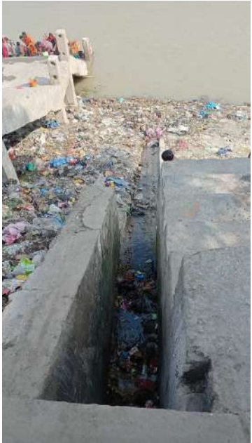
Outfall falling into Ganga
