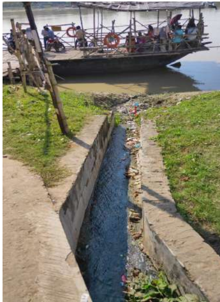
Outfall falling into Ganga
