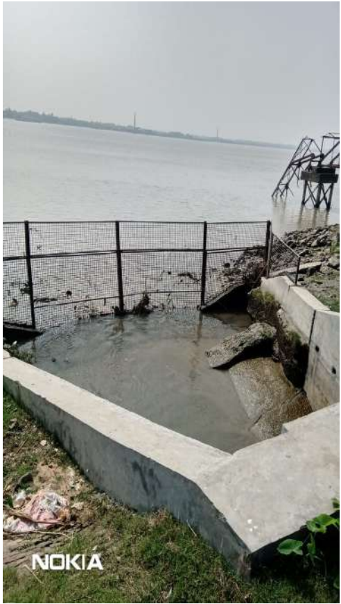
Outfall falling into Ganga
