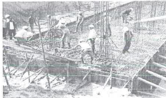
Concrete poured by pumping, placed manually using shovels and compacted using needle vibrator
