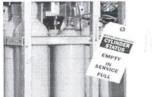
Identification of Empty cylinders
