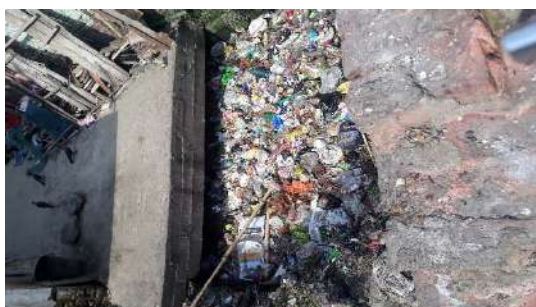
Sewage water source for BESU LS
