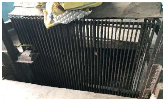
Grid Chamber at Ichapur MPS
