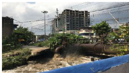
By-pass Discharge arrangement at Bagjola Canal
