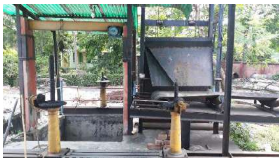
Inlet point at MPS
