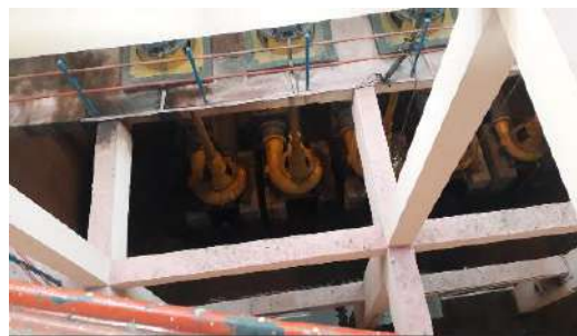
Existing Pumpsets at the MPS
