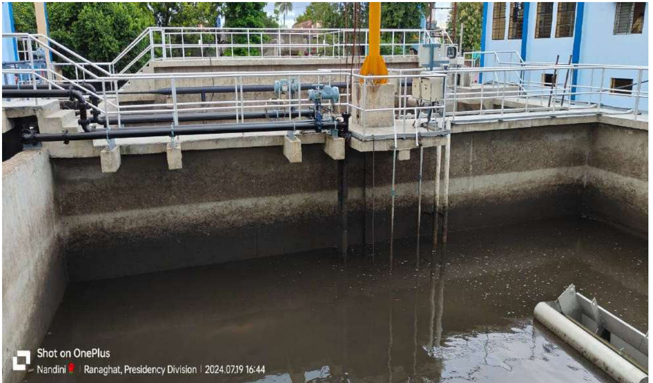
STP at Silver Jubilee Road - Ranaghat, Nadia
