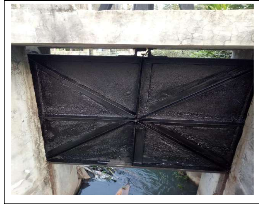
HALISAHAR DRAIN LOCKGATE
