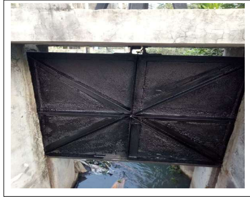
HALISAHAR DRAIN LOCKGATE
