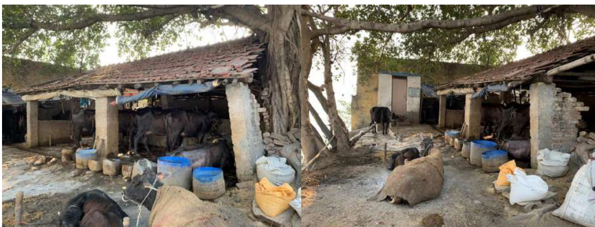
Figure 6.1 Structural Impact on Cattle Shed in Bally
